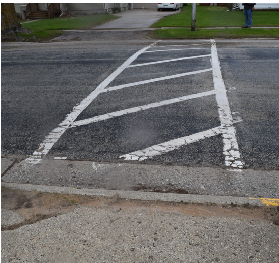
Crosswalk with no curb cuts in front of St. Paul's Evangelical Lutheran School. Source: Bay-Lake RPC, 2025
