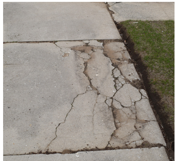
Sidewalk in need of repair on Cleveland Avenue. Source: Bay-Lake RPC, 2025
